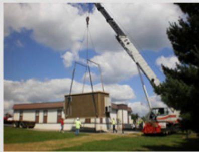
A pre-cast building to house fiber-optic cable for the Connecting Appalachia Ohio Middle Mile Consortium project is placed behind the former hospital building for Horizon by an 80-ton crane from Capital City Crane. - Photo courtesy Horizon
