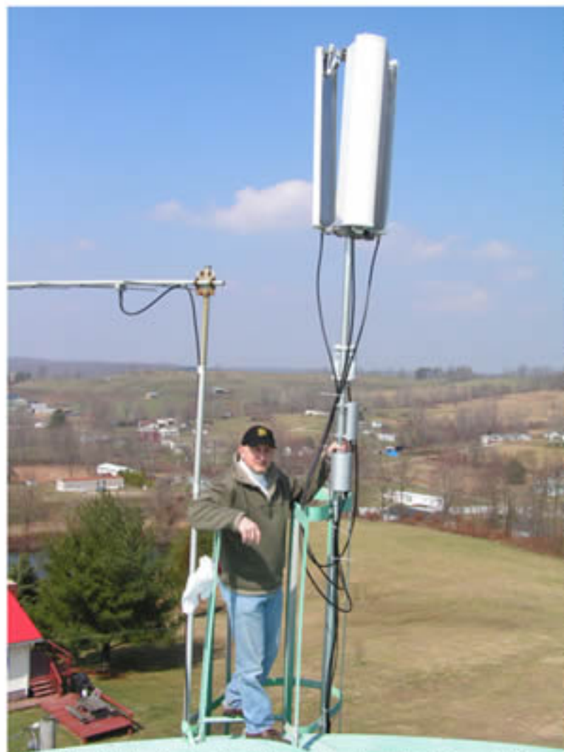
Alan Escovitz stands atop the Vinton water tower, holding on to the stand of antennas installed by the Connecting Rural Ohio team.
